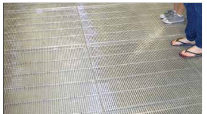
Floor grates in the main entrance will collect dirt and debris, which will make it easier to keep the building clean.
